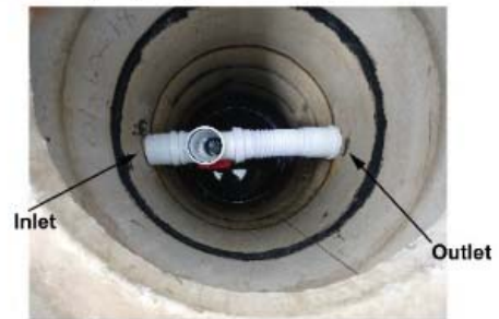
HFCW Sampling Sump
