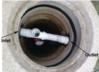
VFCW Sampling Sump
